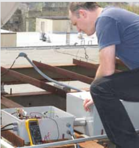
Graduate student Chris Eldridge works on rooftop solar panels at the College of Engineering complex.
